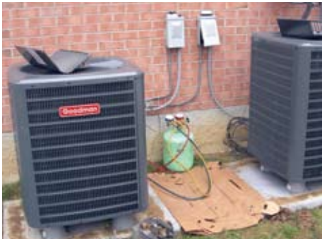
We install properly sized, energy-efficient equipment
