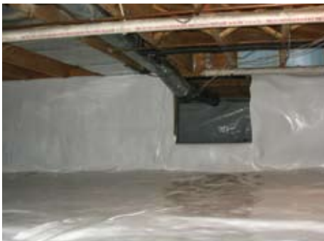
We condition crawlspaces to reduce energy losses and improve indoor air quality
